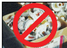
INCORRECT (Protective caps not in place)
