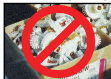
INCORRECT (Protective caps not in place)
